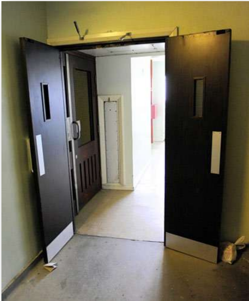
Fire doors at sister block in Camberwell Source : London Standard
